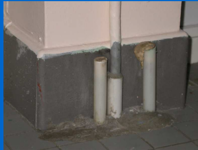
Pipes conduct air emissions towards the kids sleeping room . High levels of toluene have been highlighted.
